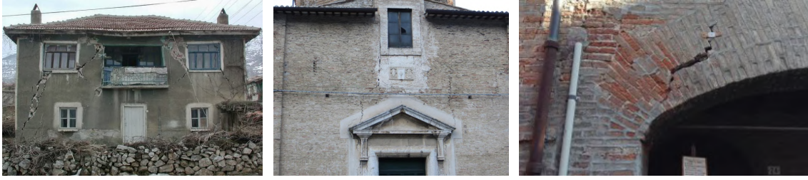
Figure 1.1: Illustrations of earthquake-induced damages on masonry structures.
