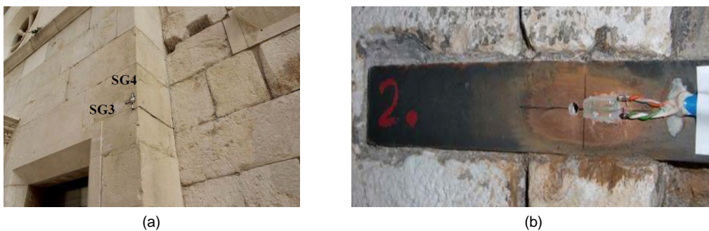
Figure 2.1: Example of using RSGs for monitoring masonry structures (Pictures by courtesy of Duvnjak et al. (2016)): (a) Overview of a measuring point; (b) Detail of a measuring point.
